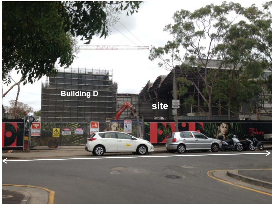
Figure 3: View of the subject site from Eve Street looking north with Building D of the Erko development in background
